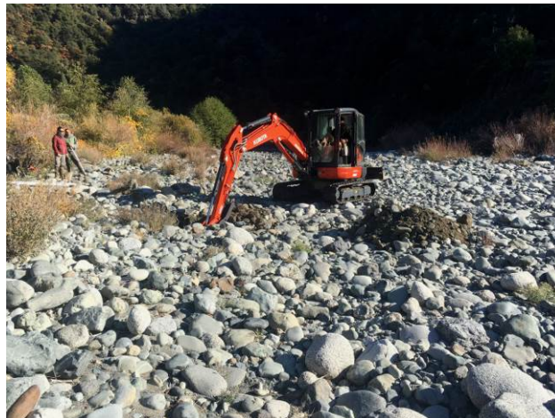
Figure 5. Photograph showing a Kubota Excavator excavating Pit 1 on the Nordheimer Confluence Bar, Salmon River Sub-Basin, California.
